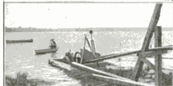
The Barge is Anchored near the Shore and Carries the Pump and Engine
