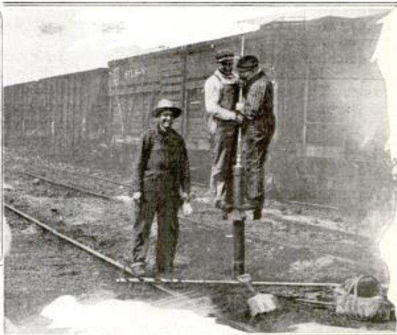
Ascertaining the Depth of a Railroad-Yard Fill: The Weight of the Two Men Gradually Forces the Casing Down into the Hole Made by the Sand Bucket. The Auger Lying on the Rails is Used to Penetrate Clay
