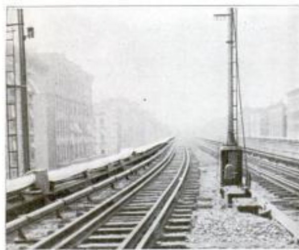
Cheesecloth Canopies Erected over the Conduits Reduced the Temperature and Prevented Recurrence of the Short-Circuiting
