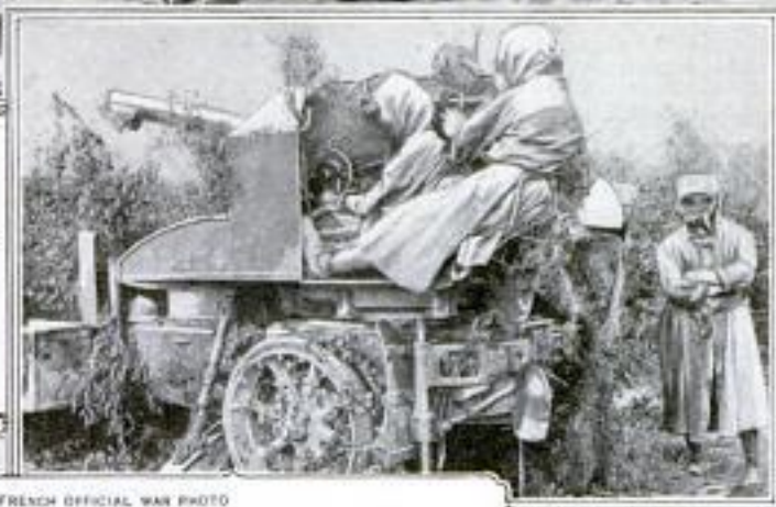
Railway Construction in the War Zone has been Reduced to a Fine Art, as is Indicated by the Photograph Presented at the Top of the Page. It will be Observed That Rail Locks are Employed Instead of Spikes, and That Track is Laid Almost as Rapidly as the Ties can be Distributed and Alined. The Supply Train Follows the Workmen as the Rails are Projected. The Picture was Taken in the Aisne District
