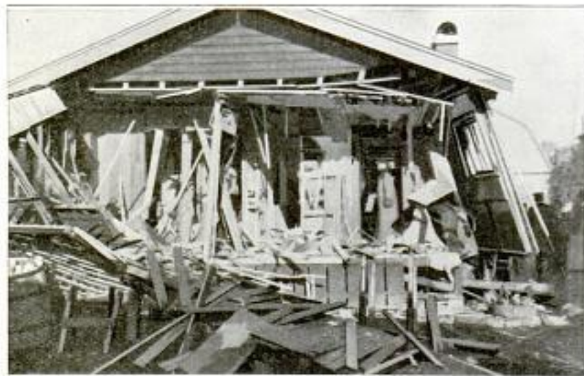
Bungalow Wrecked by Explosion of Water Heater, Caused by Failure to Shut off the Gas
