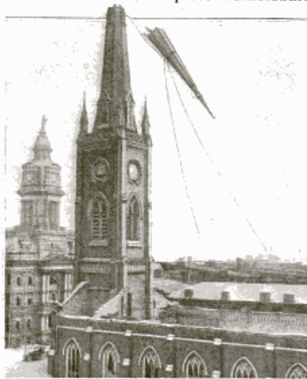
Unusual Photograph Taken at the Instant the Point of This 205-Foot Church Spire was Toppling to the Ground
