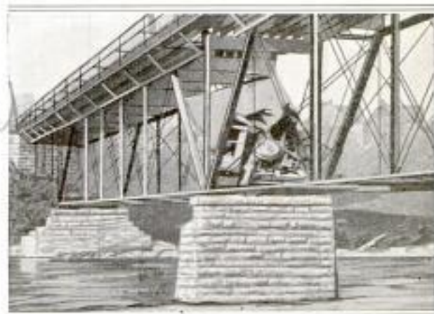
Bridge After It Gave Way under Heavily Laden Truck: The View Shows the Strange Manner in Which the Timbers and Pier Caught the Vehicle and Prevented It from Falling into the Water
