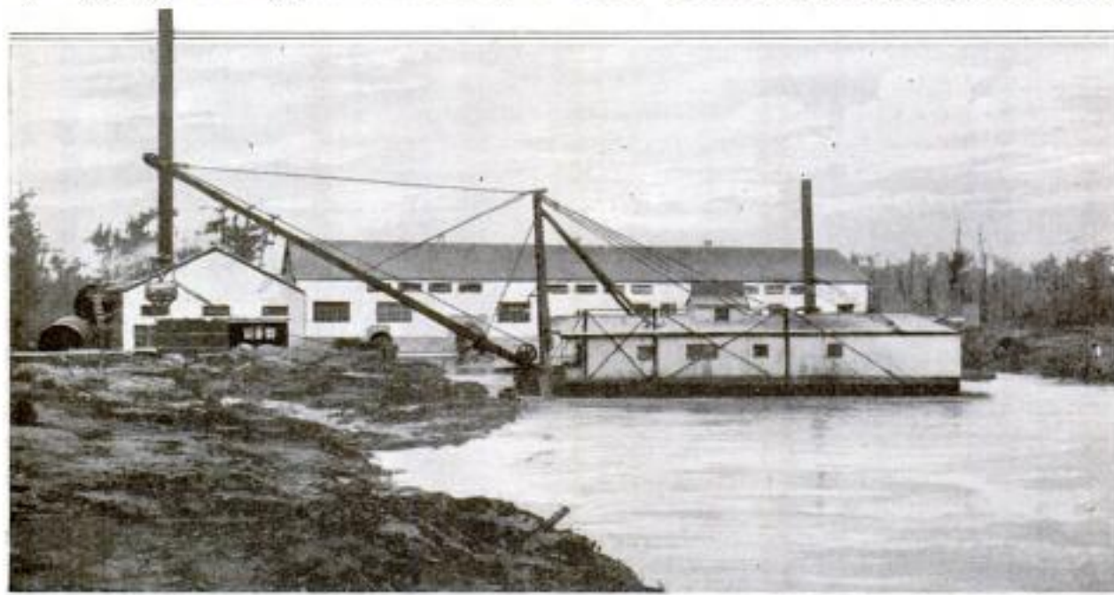
Dredge at Work Deepening One of the Big Irrigating Canals in Southern Louisiana Where the Reclamation of Swamp Lands is being Carried Out: The Building in the Background Is the Pumping Station for the District
