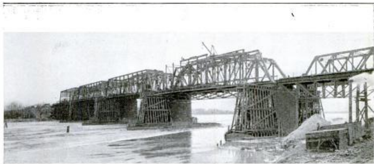
Showing Operations in Progress before Flood Time: The Old Superstructure is Supported on Temporary Piers and by Trusses Anchored to the New Bridge
