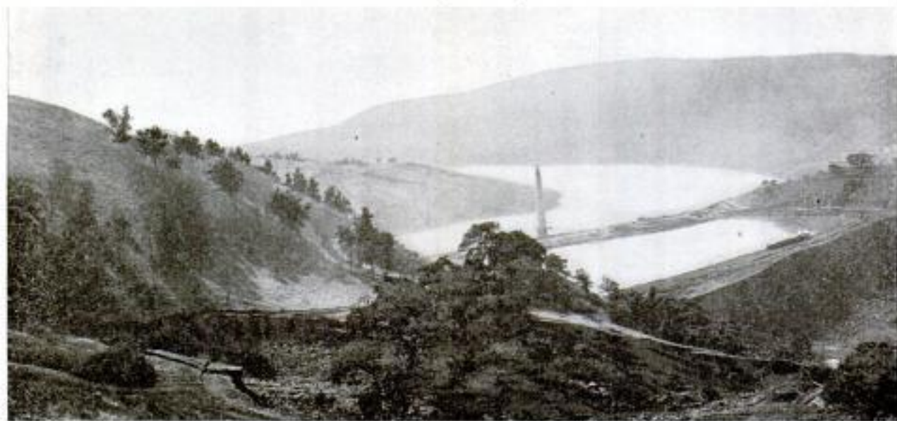
Panorama of the Calaveras Dam, Now under Construction near San Francisco, Which will More Than Double the Width at the Base, 1,300 Feet. Steam-Shovel Operations are Shown, also the
