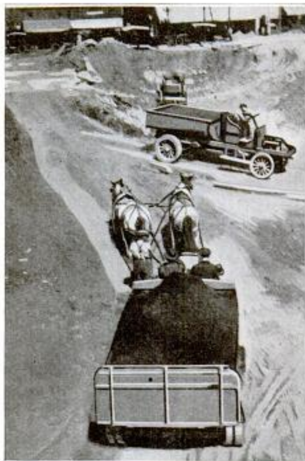
The Team Shown Here was Regularly Employed in Helping Six-Ton Motor Trucks Make the Steep Ascent from the Bottom of This Excavation to the Street Level
