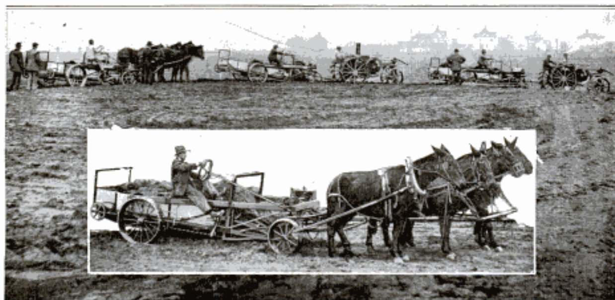
The Self-Loading Excavator, Which Peels Up One and Three-Quarters Cubic Yards of Dirt in About 20 Seconds, is Said to Reduce the Cost of Road Grading, Making Cuts and Fills, and Doing Similar Work, Nearly Two-Thirds. A Battery of the Machines in Use, and a Close View of One of Them, Appear Above
