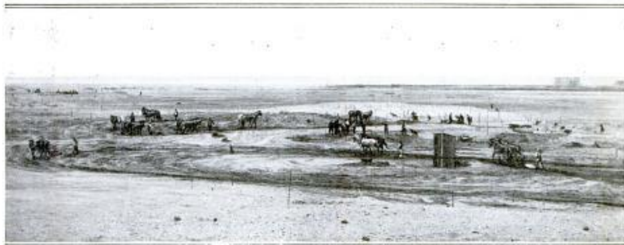
Leveling with Scrapers After the Filling-In had been Completed: This View Gives a Good Idea of the Large Scale on Which the Operations were Conducted
