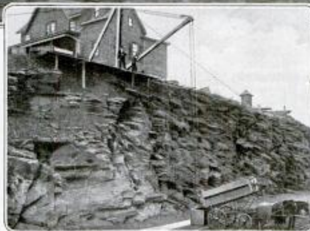
PHOTOS COPYRIGHT, BROWN & DAWSON The Architect's Drawing Reproduced at the Top Shows the Big Movie Plant as It will Appear When Construction is Completed. The Lower Picture Gives a Glimpse of the Block of Ground Left High in the Air by Street Graders and Shows the Difficulty Encountered at the Outset in Getting Fuel and Other Materials to Residences Above
