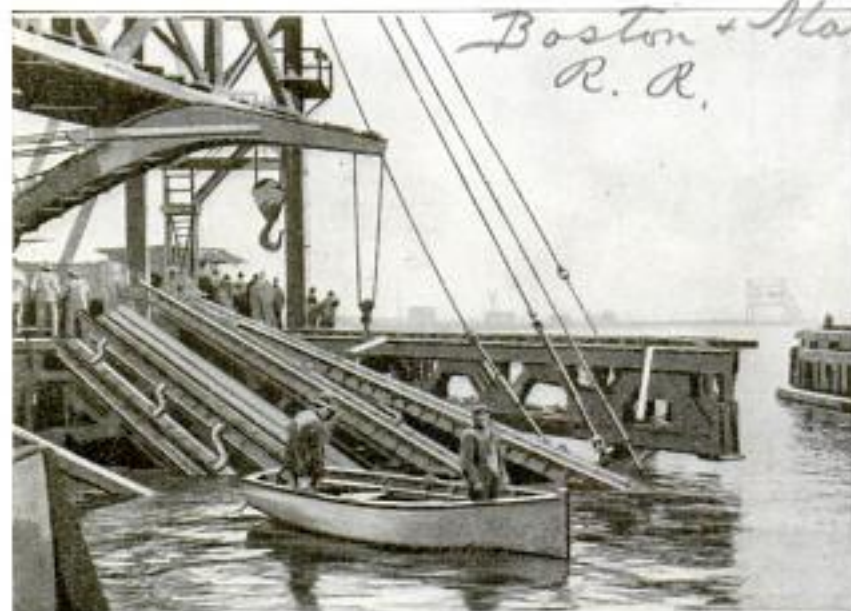
Railroad Drawbridge over Mystic River near Boston. Wrecked by the Snapping of the Cables of Two Spans: The Third Span, the Most Distant One Shown Here, was Utilized as Soon as Possible in Relieving Traffic Congestion
