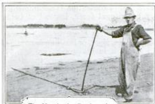
The Man in the Rowboat is Laying the Cable in a Loop Extending Out into the Lake. One End being Held Fast on Shore by Means of the Rod
