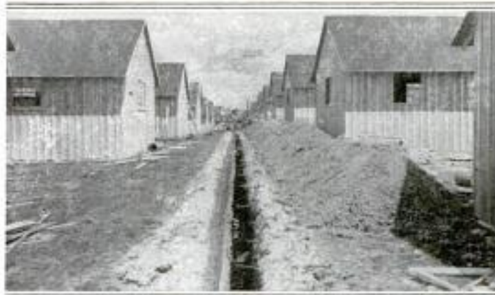
Looking down the Street Separating the Bathhouses from One Row of Barracks and Showing a Trenching Machine at Work Cutting a Ditch for a Sewer Conduit: At the Time the Picture was Taken All of the Buildings were Nearing Completion
