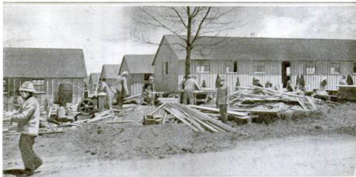
If This Picture could Talk, It would Scream, for It Shows One of the Power-Driven Saws That Shrieked from Morning until Night for 10 Days. Standing in the Foreground near the Middle Is Lieutenant James H. Reding, One of the Ohio Engineers Who Assisted in Supervising the Work
