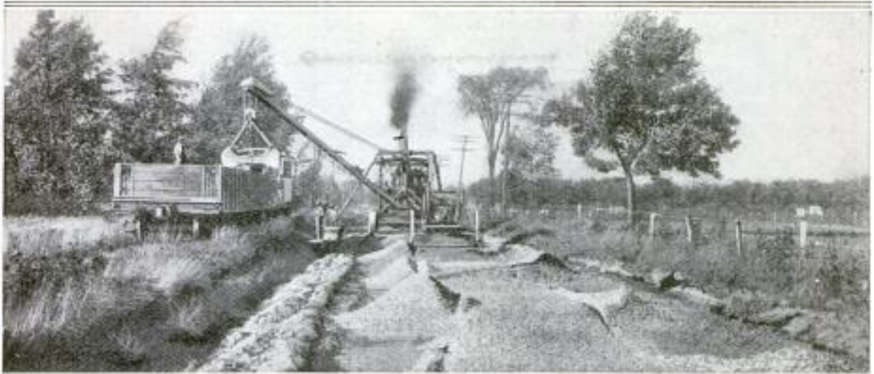
Spreading Crushed Stone with a Minimum of Manual Labor: The Gravel Car and a Self-Propelling Crane Move Along Side by Side, While the Stone is Deposited in Piles, and Spread by a Scraper
