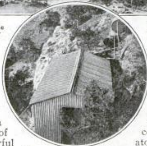
Power House in the Cañon That Furnishes Electric Light for the Movies, 50 Feet Above
