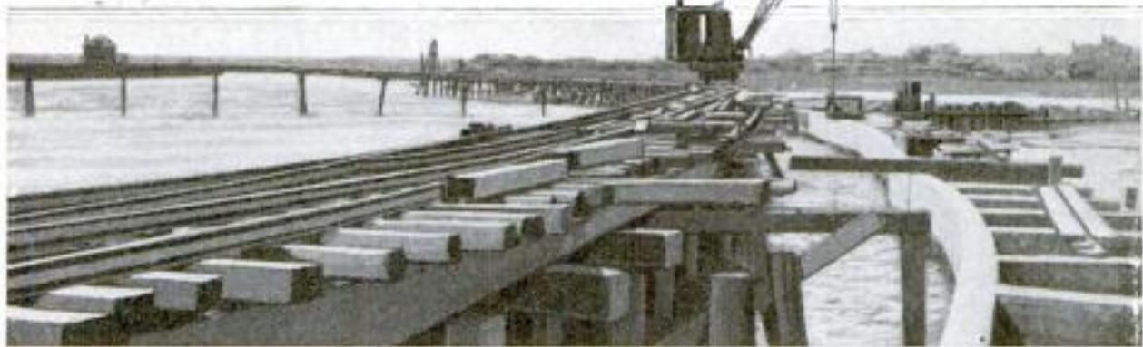
North Wall of the New Concrete Inlet to Shark River. Showing the Trestle Used in Placing Reinforced-Concrete Piles Made at a Special Plant Set Up on the Neighboring Shore
