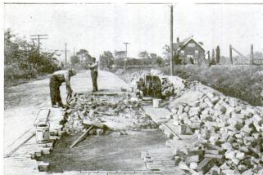
Cleaning Out the Old Mortar to Patch Brick Pavement in Cleveland: A Pneumatic Chisel is Used, with Power Furnished by the Air Compressor alongside the Patch, and One Man can Do the Work of Three with Hatchets
