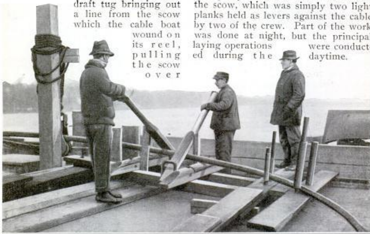
Method of Controlling the Movement of the Cable as It Dropped to the River Bed
