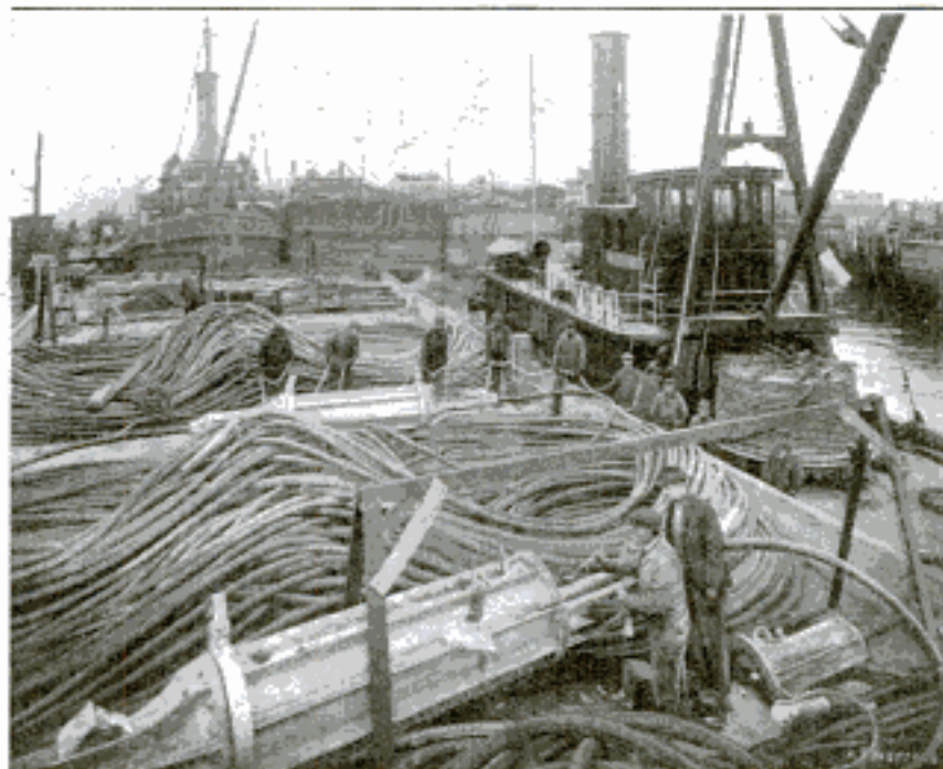
Getting the Nyack-Tarrytown Telephone Cable Ready for Laying beneath the Waters of the Hudson River: Most of the Cable Lies on a Scow, with the Loading Pots in the Foreground
