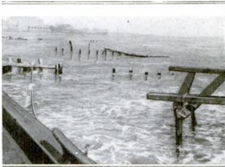
Remains of Wooden Jetties Built to Protect the Inlet to the Shark River on the New Jersey Coast. Showing What the Sea has Done to Them: The State is Now Building a Concrete Inlet Mouth
