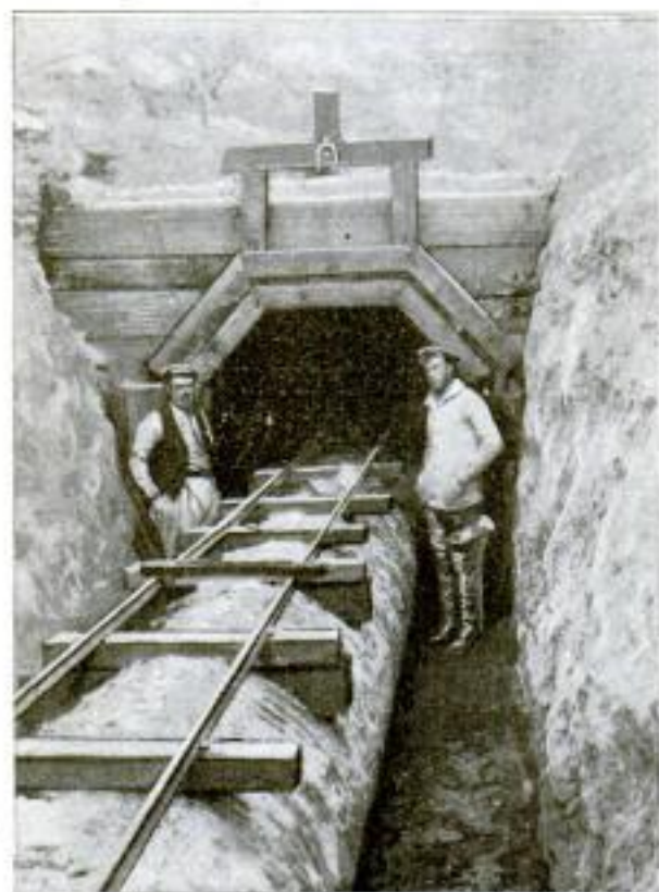
More than a Mile of Tunnels was Cleaned Out by the Aid of a Small Dump Car Run on This Track with Its Pipe-Line Roadbed
