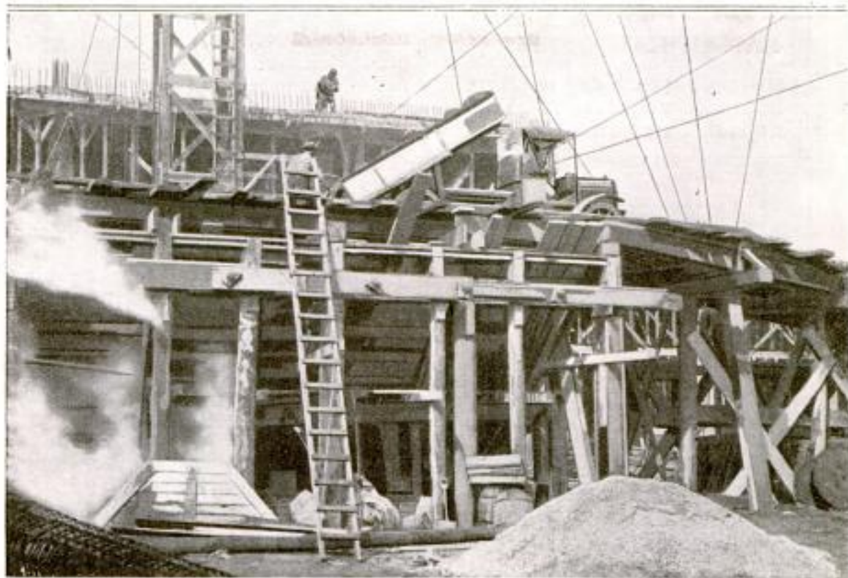
Platform on Second-Story Level from Which Trucks Dumped Their Contents into a Bin Below, Thereby Saving Much Labor in the Handling of Building Materials for a $500,000 Concrete Structure
