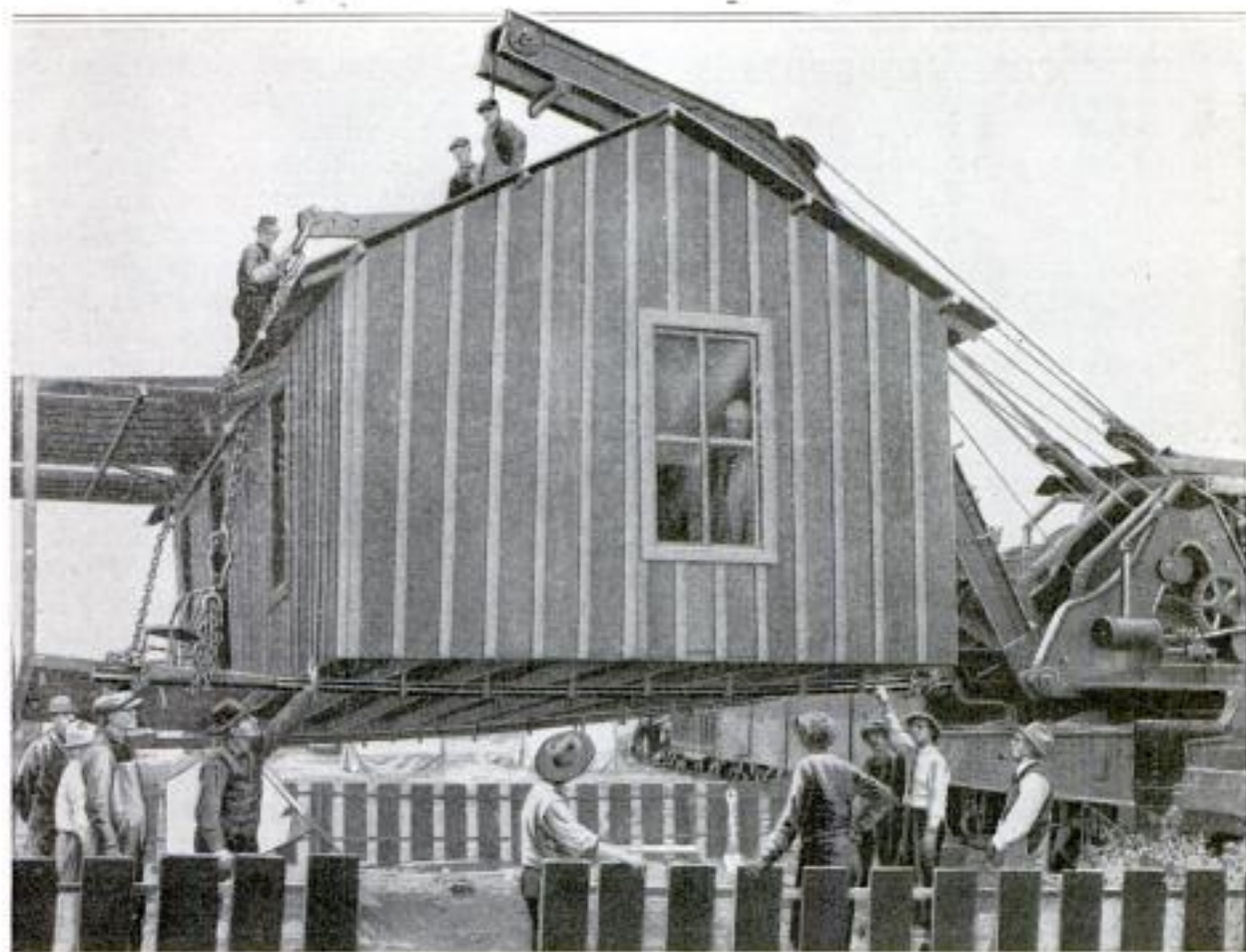
Moving a House with a Railroad Derrick: The Building was Supported on Steel Rails, Attached by Chains to the Arms of the Derrick. The Man at the Window and Other Residents were Undisturbed
