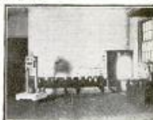
Battery Charging room, showing lighted switchboard and distilled water rack.
