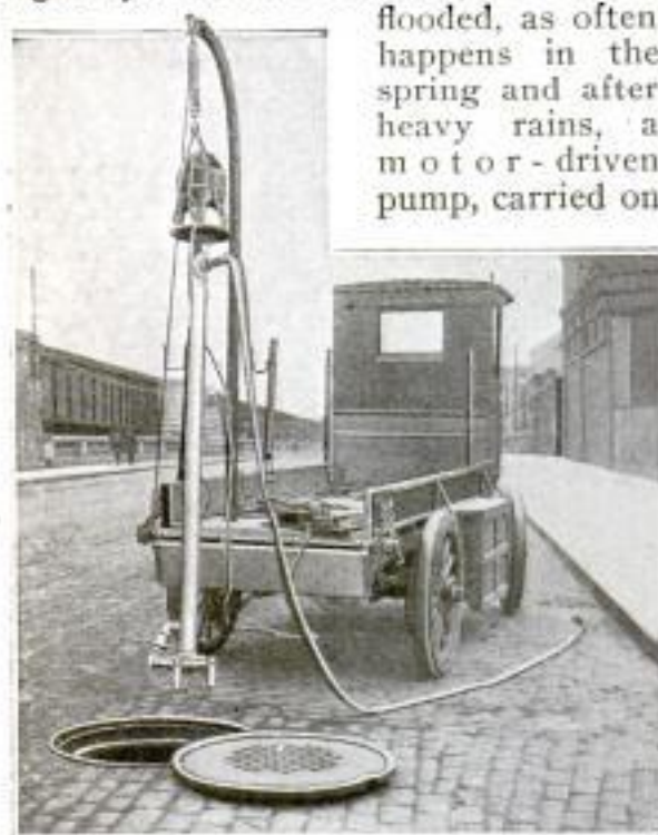
Pump in Position to be Lowered into a Flooded Manhole: An Electric Motor at the Top of the Upright Pipe Runs the Small Pump at the Bottom
