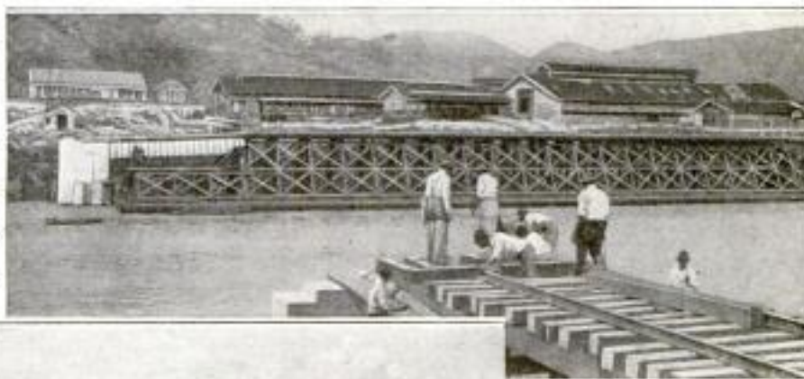
The Picture Above, Taken While the Construction Work Was Still in Progress, Shows the Long Pontoon and Trestle Drawn along One Side of the Canal
