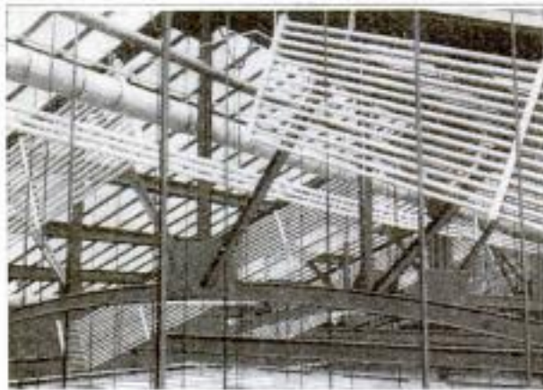
A Portion of the Loft under the Glass Roof, Showing the Radiators Which Are Part of the Novel Heating System
