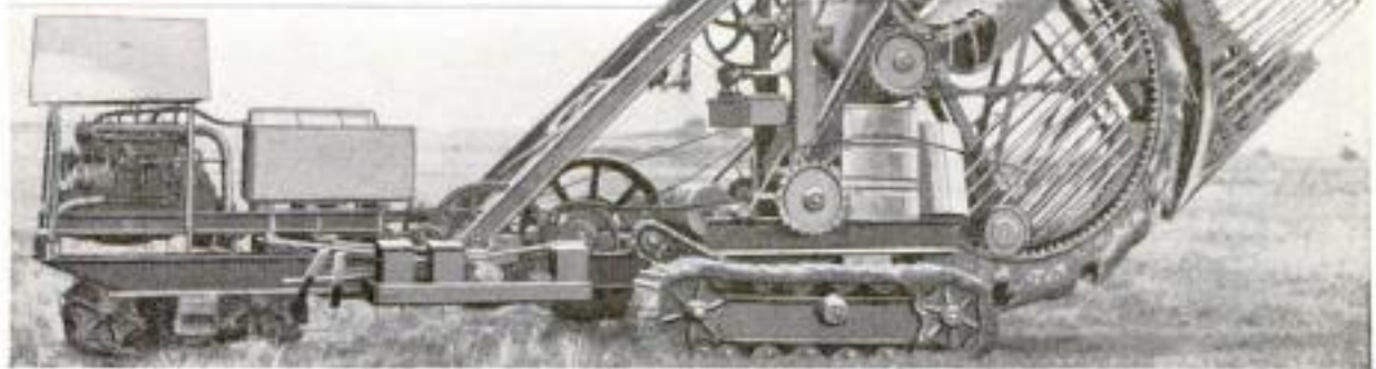
Big Ditching Engines of This American Type are Used by the Germans in Constructing Intrenchments along the Various Battle Fronts
