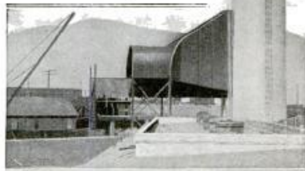
This Chimney Rises 300 Feet into the Air at a Texas Smelter, and was Built of Concrete with Adjustable Steel Forms. The Platforms Seen Part Way Up Furnish Means for Testing the Inside Temperature and the Volume of Smoke
