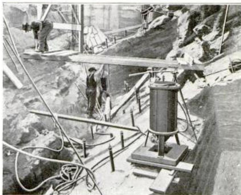
In the Center of This Picture Workmen are Seen Applying a Water-Pressure Test to the Granite-Ledge Foundation for a Big Dam, before Forcing a Cement Grout into the Drill Holes, to Fill Seams and Fissures through the Two-Inch Pipes Seen in the Holes
