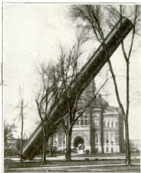
After One Side of the Foundation had been Removed, a Steady Pull on a Cable Attached near the Top of the Structure Caused the 110-Foot Standpipe to Crash into the Street
