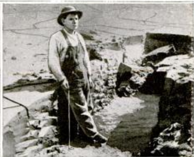
View of One of the Emptied Settling Basins, Showing a Deposit of 30 Inches of Silt Which Accumulated in One Year
