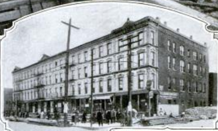
Here the Same Block as Above is Seen Soon After It Began Its Backward Journey to a New Site in the Rear. The Jackscrews Are in Place below the Sidewalk Level, and Interested Spectators are Watching the Workmen
