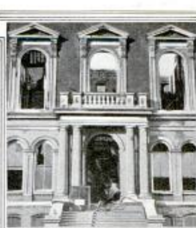
View of Main Entrance After the Roof Collapsed. The Line of Hose Seen on the Steps was Cut by Falling Debris
