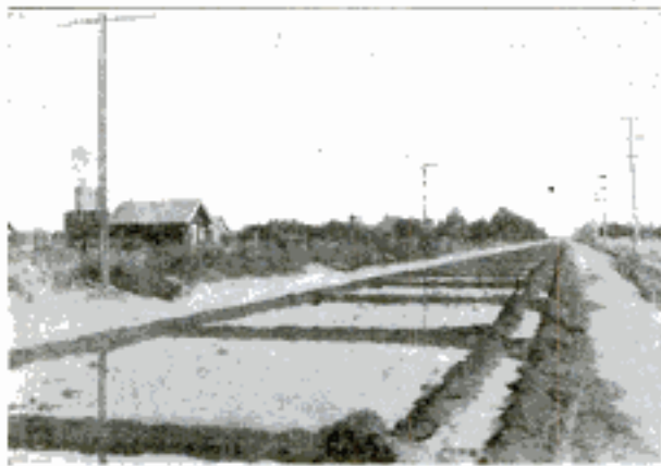
By Making Double Dikes near the Edges of This Newly Laid Concrete Pavement, Less Water was Required to Cover the Curved Surface than if a Single Dike had been Made
