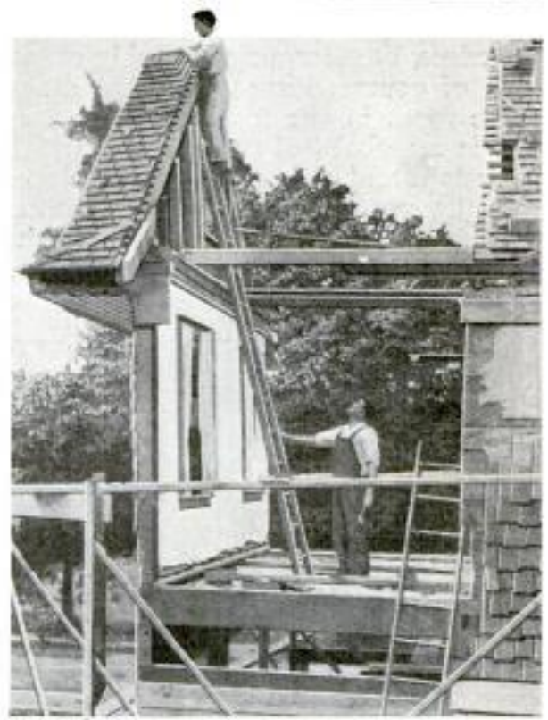
Wing of a House Which was Enlarged by Cutting Off the End and Moving It Out on String Pieces with a Rope and Crowbars, After Which the Intervening Space was Walled In
