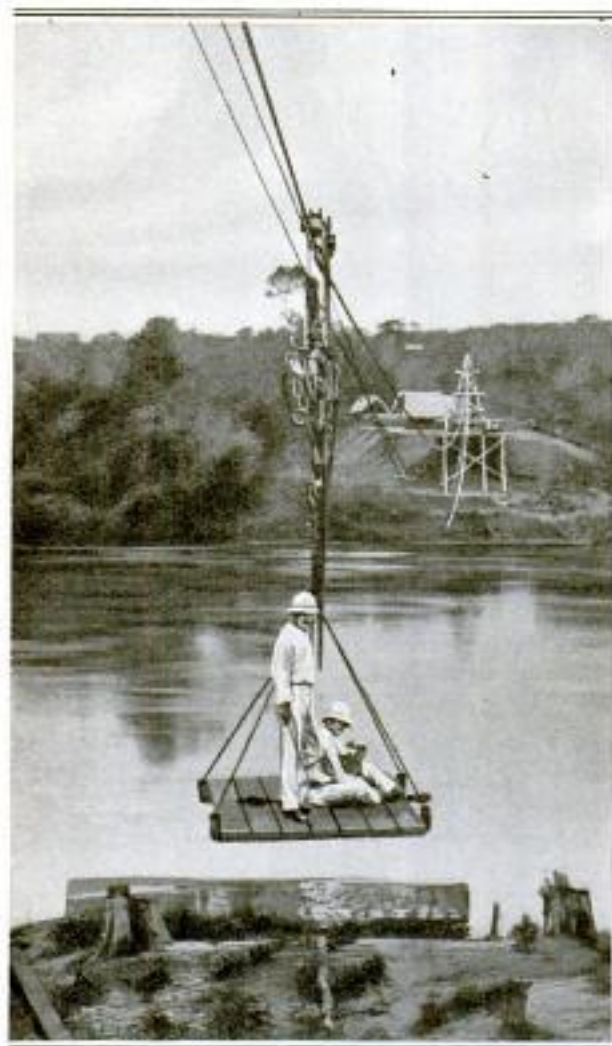
Preparing to Build a Temporary Military Bridge across a Stream in Western Africa: The Ropeway Serves for Transporting both Men and Materials
