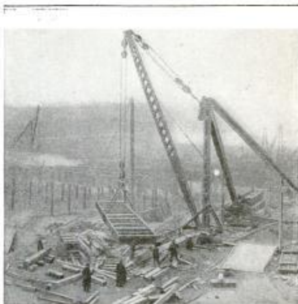
Fig. 3. Seventy-Five Ton Girder Handled by Steel Derrick: Twenty-One Parts of Line are Used with Double Blocks in the Load and the Boom Lifts
