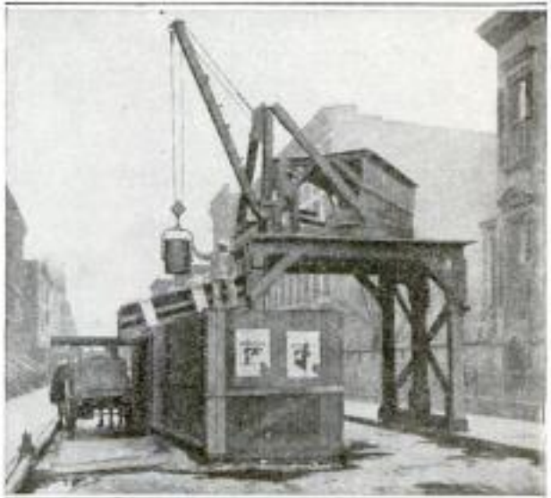
Fig. 2. Handling Dirt from a Tunnel Excavation: The Use of a Platform and the Tip Bucket Are Suggestive
