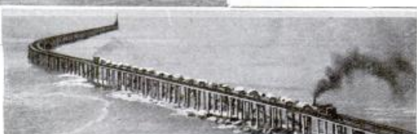
Trainload of Stone being Hauled over Trestle during Construction of North Breakwater. With These Structures and Dredges, a Deep Channel is being Provided into the River
