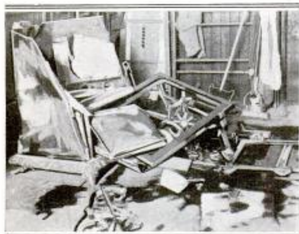
A Kitchen Stove Which was Wrecked by the Explosion of Gas Which had Escaped through an Open, Unlighted Burner for Several Hours
