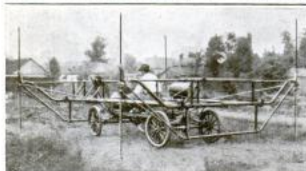
The Driver of the Machine can Bore Four Holes at Once with This Device, Then Withdraw the Augers from the Earth, and Move on to a New Position without Leaving His Seat
