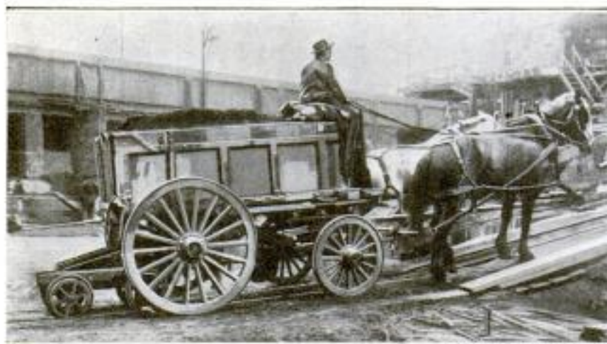
With This Barney, Drawn by a Hoisting Engine, It Was Possible to Haul Full Loads Out of a Foundation Pit without Extra Horses
