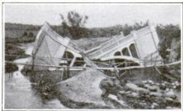
A Reinforced-Concrete Bridge in the Philippines as It Appeared after a Recent Typhoon
