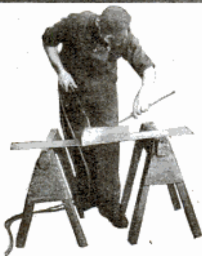
Welding two pieces of angle iron by oxy-acetylene process. Final work has neat finish and great strength.
