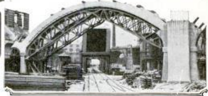
One of the Concrete Arches Showing the Temporary Steelwork Still in Place
