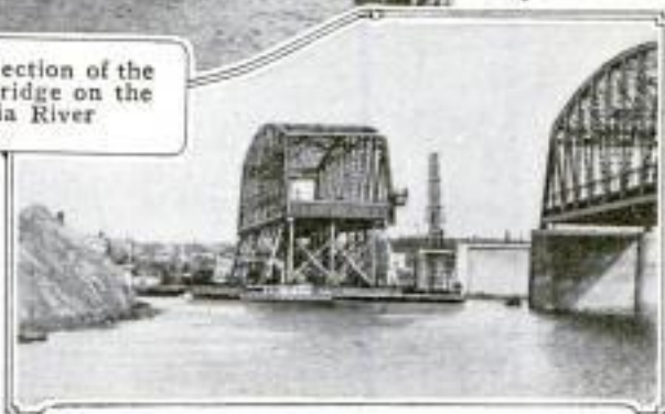
One of the Steel Sections, Weighing More Than 400 Tons, Almost in Its Final Position in the Bridge
