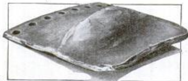
Mud Which Accumulated in a Boiler Caused a Portion of Its Shell to Become Red-Hot. The Pressure within Produced This "Bag," Which Projects Eight Inches
