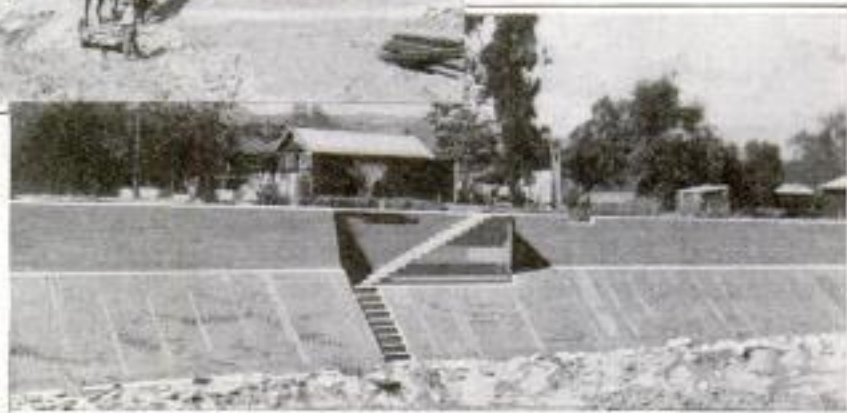
Showing a Section of the Completed Concrete Wall Which will Confine the Arroyo Seco River to Its Channel; Also the Method of Erecting Forms for the Work
