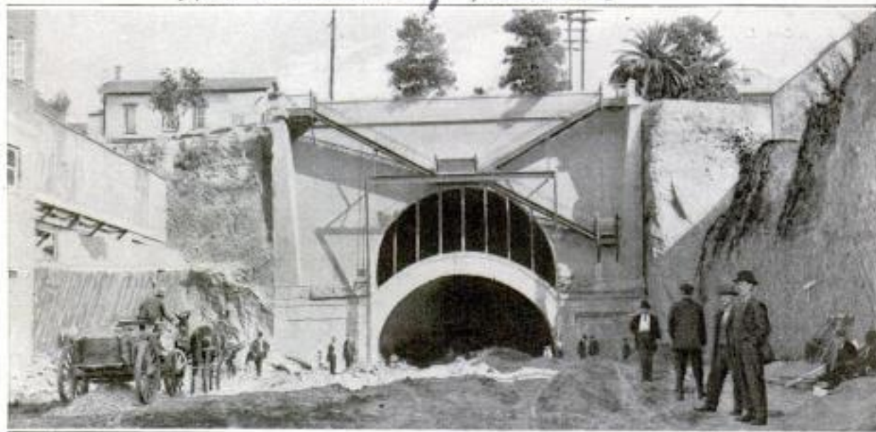
This Photograph Gives a Clear Idea of the Method of Construction Followed in Correcting the Grade of the Tunnel to Correspond with the New Street Level
