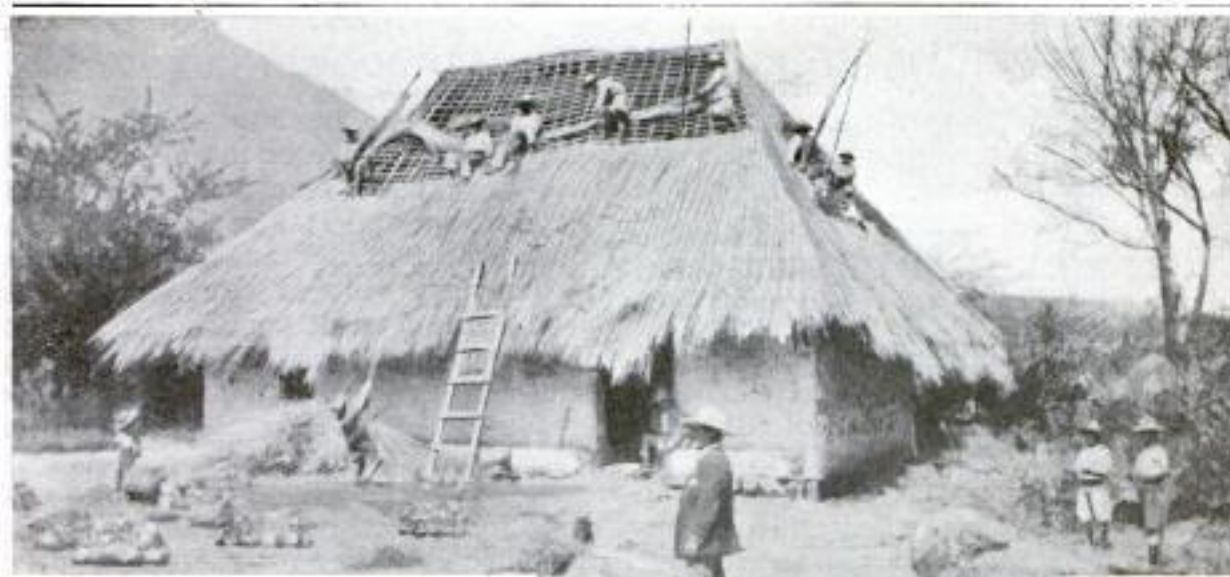
The Fine Residence of a Wealthy Guatemalan Sugar Raiser in Process of Construction. The Round Balls in Front of the House Are Heaps of Raw Brown Sugar Ready to be Carried on the Backs of Natives to a Refinery Perhaps a Hundred Miles or So Away
