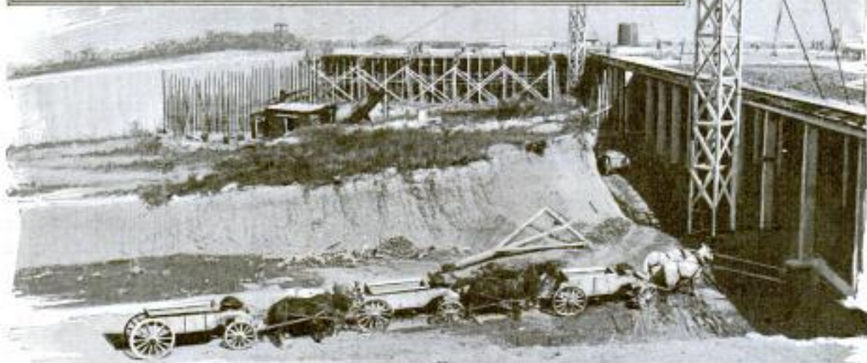
The Basin When Finished will Hold More than 20,000,000 Gallons of Water. It is Situated on a Hill 250 Feet above the Lowest Part of the City. This Shows It Half Completed
