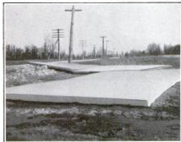
A Recent Ohio River Flood Carried These 20-Ton Slabs 30 Feet Out of Line
