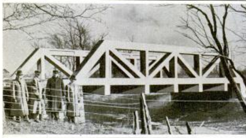
This Bridge, Formerly an Old, Unsafe Steel Structure, was Made Serviceable by Coating It with Concrete
