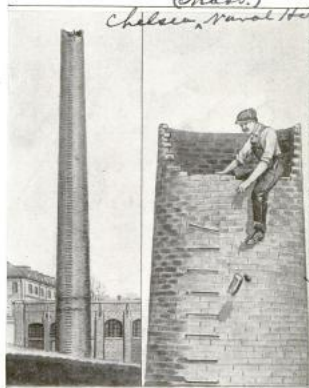
Marooned at the Top of This Chimney, a Workman Saved Himself by Removing the Bricks and Cutting His Way Ten Feet to the Iron Ladder
