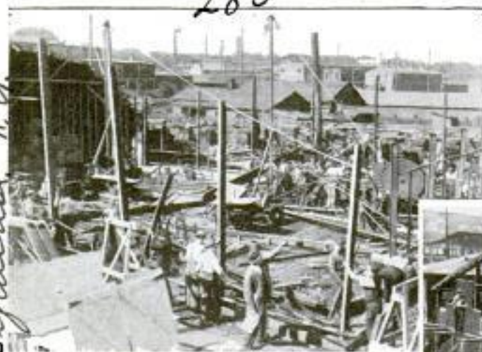
This Photograph was Taken at 8:15 in the Morning, a Quarter of an Hour After the Work had been Started
