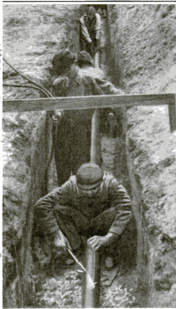
Welding the Joints of a Gas Main by Means of the Oxyacetylene Torch, with Soft-Steel Wire as the Welding Material
