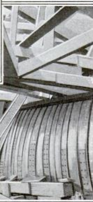
How the Steel-Sheet Piling was Bulged Inward under the Pressure of the Mud and Water
