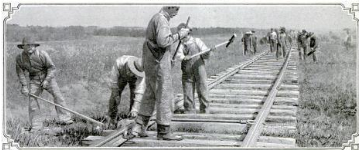
Gauging a Freshly Laid Track Projected across a Stretch of Open, Flat Country Where Grading was Dispensed With
