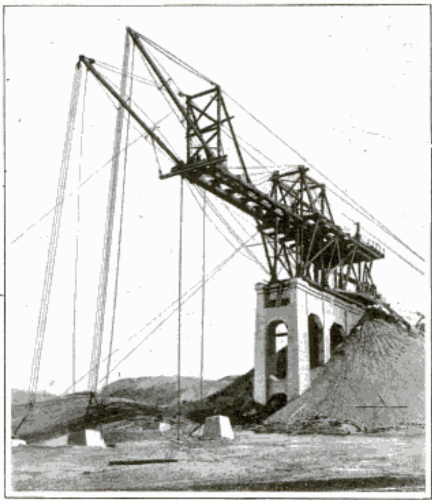
The Wooden Cantilever Traveler in Use Beginning the Erection of the Viaduct
