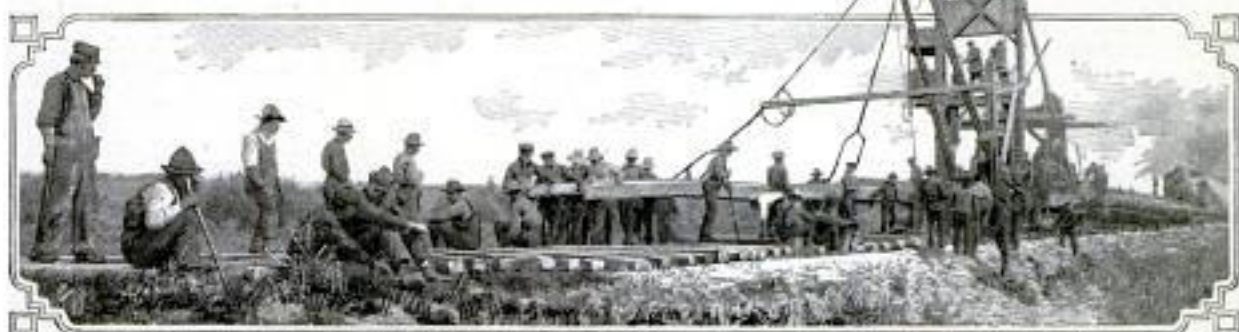
Here a Track Layer is Engaged in Pushing Rails Ahead along the Newly Placed Ties Extending in Advance of It
