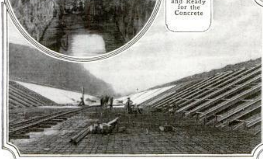
Steel Reinforcing in Place for Concrete Walls and Bottom; This Is One of the Points Where the Lava Rock Is Too Porous to Hold the Water
