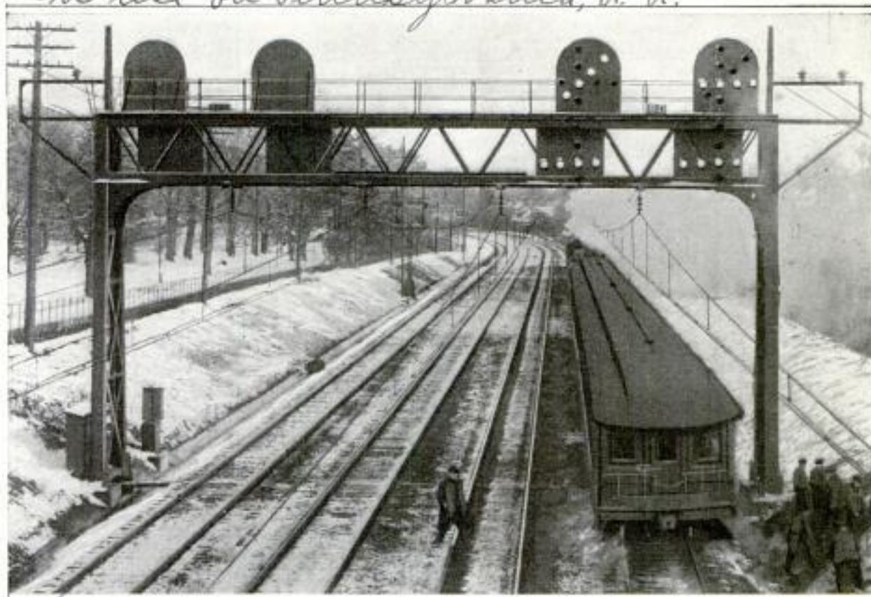
New System of Block Signals in Which Rows of Electric Lights are Employed for Giving the Standard Semaphore Indications
