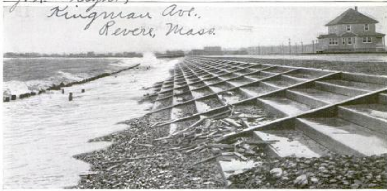
This Sea Wall, Just Completed at Point of Pines, near Boston, is Built as a Series of Steps with the Idea of Breaking the Force of the Waves
