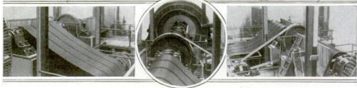
Chain Drive Placed in Service at a Hydroelectric Power Plant in Oregon: The 3,600-Kilowatt Generator is Driven by Four Chain Belts, Each 21 Inches Wide
