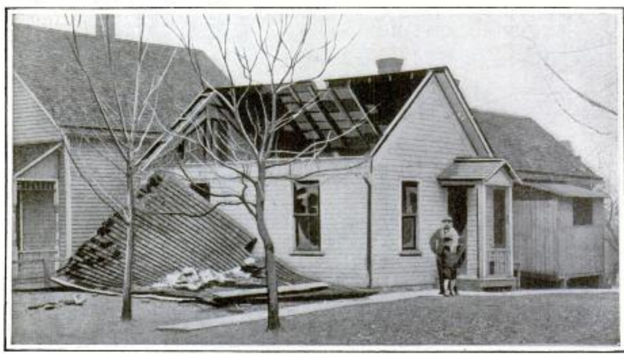
The Roof of This House was Blown Off by an Explosion of Illuminating Gas Which did Not Injure Those in the Room in Which It Occurred
