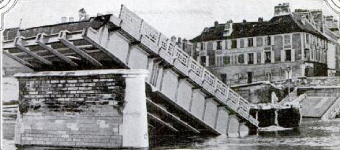
Tangled Wreckage of a Steel Bridge at Lagny, Less Than a Half Hour by Rail from Paris
