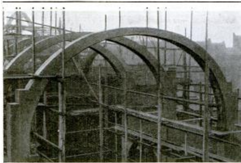
The Reinforced-Concrete Arches of a German Cathedral After the Forms were Removed
