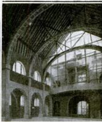
Interior of the Church Showing the Arches After the Roof had been Built
