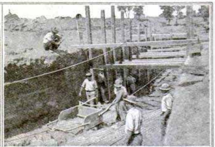
The End of the Trench: The Bucket is Provided with Handles by Which Two Men Guide It in Digging as They would a Plow
