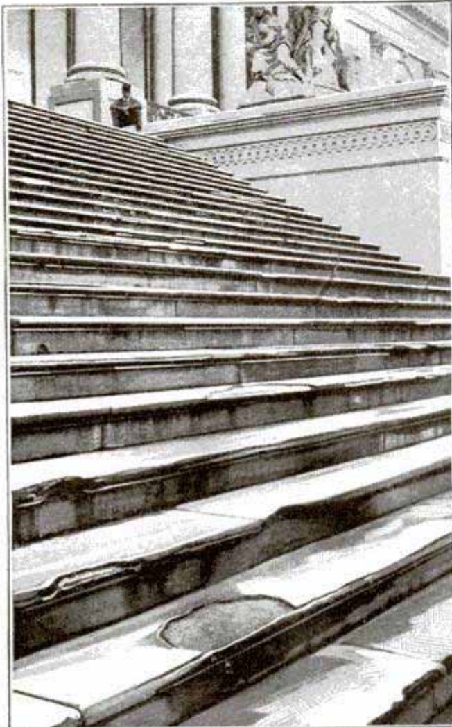
The Battered Steps at the East Entrance of the United States Capitol Which are to be Replaced After More Than 80 Years' Service
