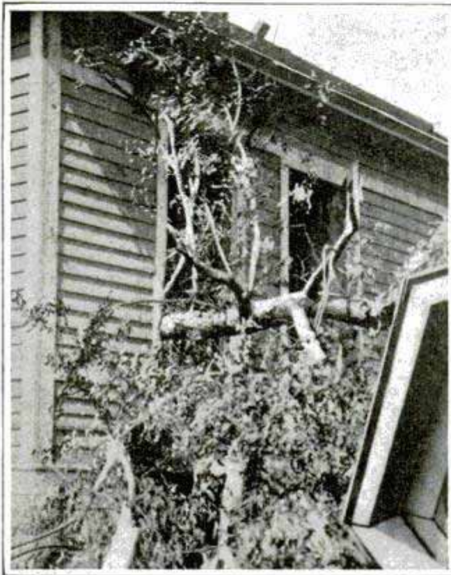
A Tree with Wide Root Spread Tossed through a Window without Injuring Casing
