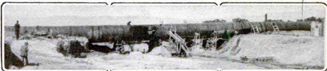
The Concrete Supports Carrying the Siphon were Destroyed by Flood, Permitting the Pipe to Fall into Stream
