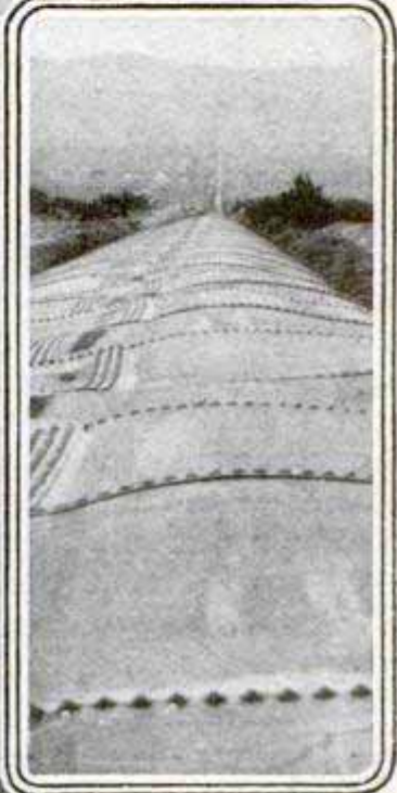
The Siphon Partly Restored to Its Original Shape by Hydraulic Pressure
