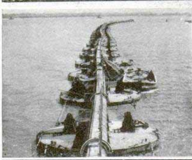
Pipe Line Used with the Hydraulic Dredge in Restoring the Old Channel
