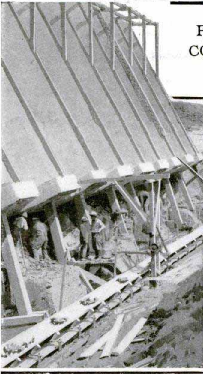
Starting the Dangerous Work of Driving Tunnels under the Sunken Elevator: From the Bottoms of Tunnels Shafts will be Sunk for the New Concrete Piers
