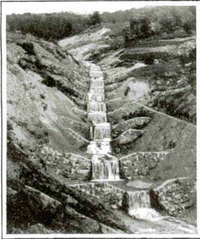
A Watercourse in the Alps, in Which Erosion is Reduced by a Series of Small Masonry Dams
