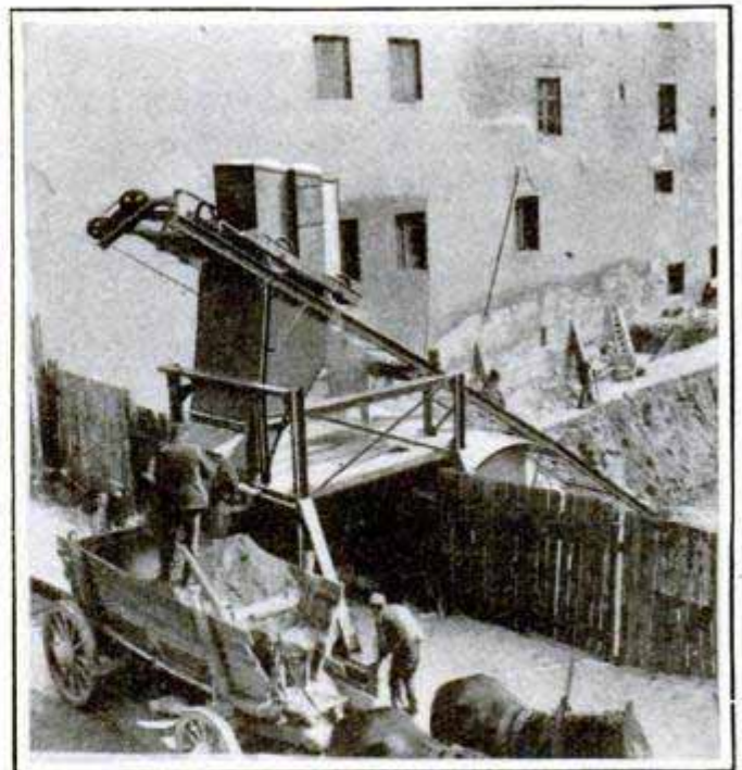
Photo by Paul Thompson Mechanical System for Hoisting Excavated Material from Basement of Proposed Building
