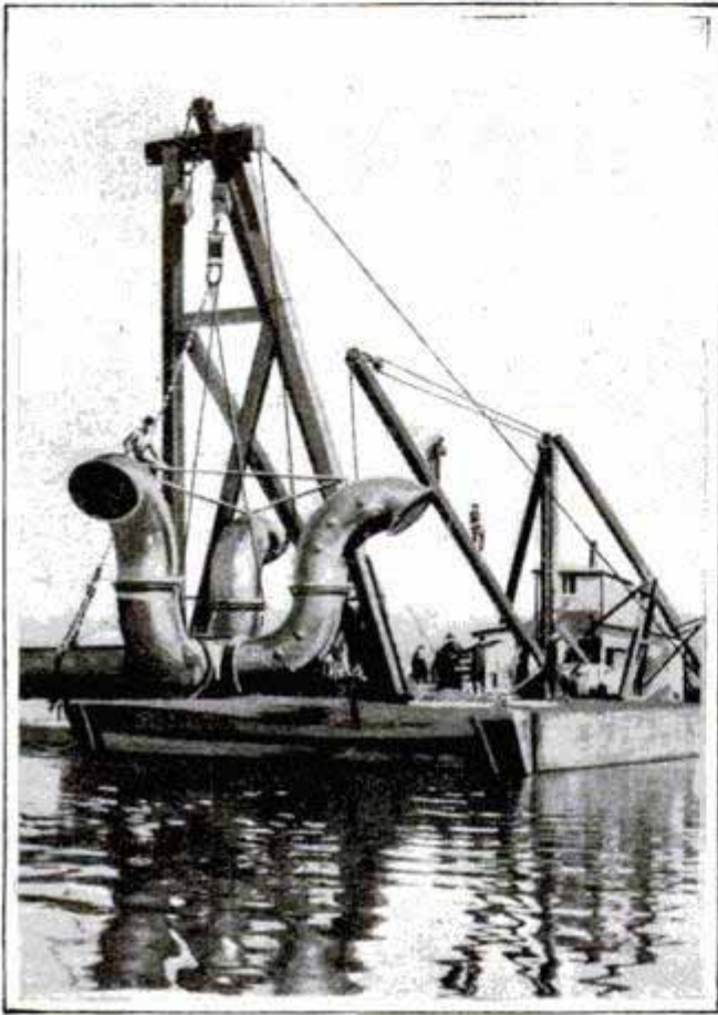
Completed Intake for Marquette, Mich., Water-Supply Main: Intake on Scow Ready to be Lowered by Derrick into Final Position
