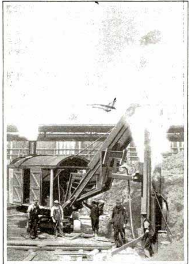
Small Steam Shovel Converted into Pile Driver for Working in Crowded Space
