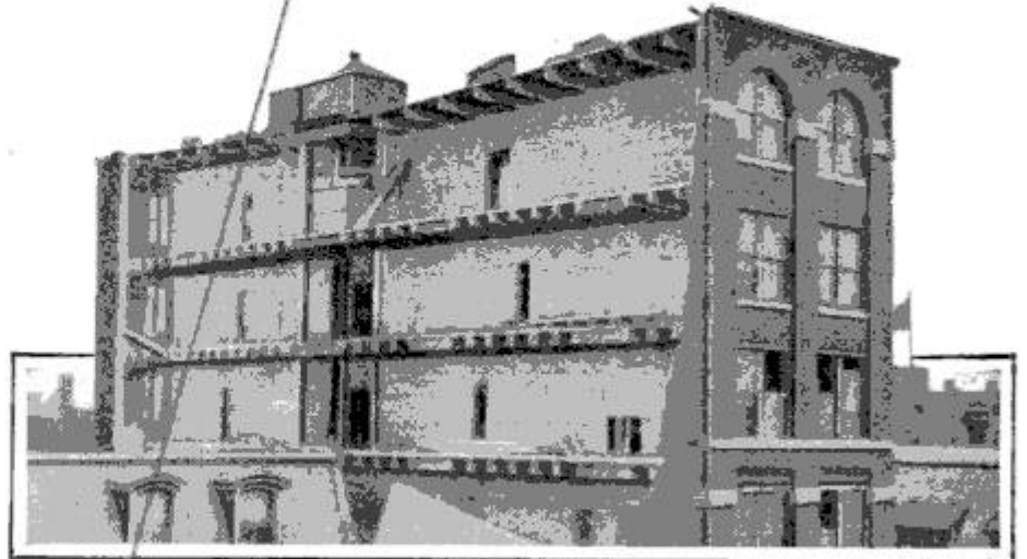
A Building Resting on Its End Walls and Jack-Screw Supports While Its Side Walls are being Wrecked and Replaced
