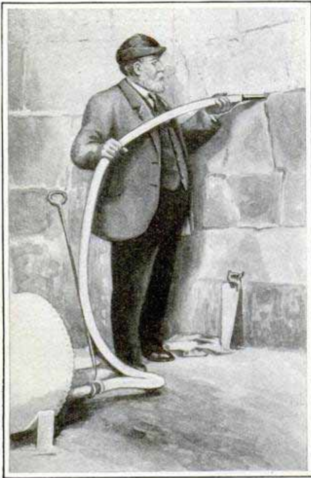
Compressed-Air Machine Forcing Cement into the Cracks in St. Paul's Cathedral Walls
