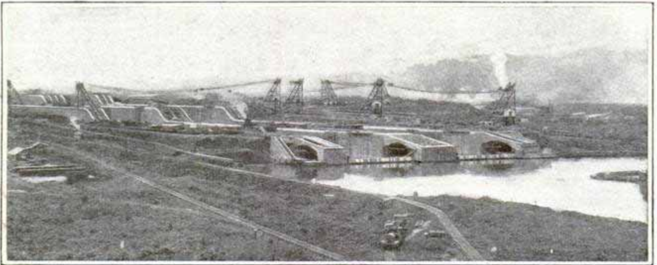
View of the Nearly Completed Gatun Locks, Which Gives a Good Idea of Final Appearance
