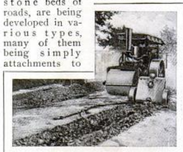
Novel Type of Machine Attached to Road Roller, to Tear Up Old Roadbed Preliminary to Resurfacing
