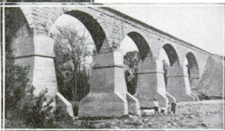
After the Steel Bands Had Been Placed and Concrete Built Up around Each Pier
