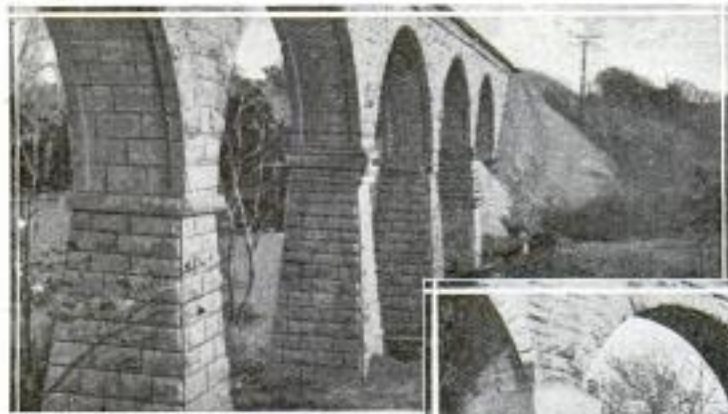
Stone Arch Bridge on Chicago & Alton Railroad before Repairs.
