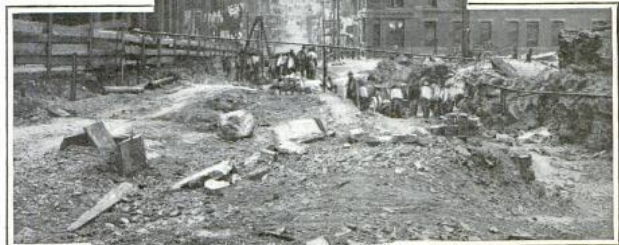
Looking Down from Grant Street, Where It was Necessary to Blast Tons of Rock
