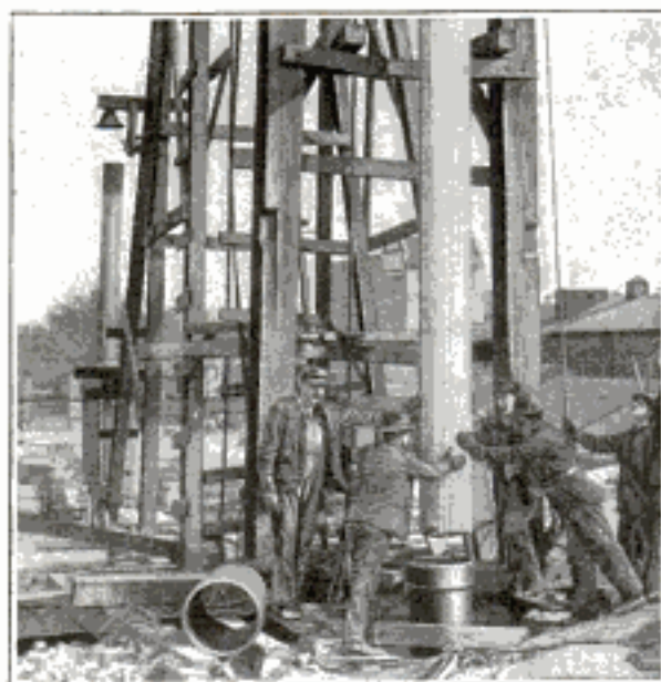
Lowering the Concrete Pile into Steel Bore, a Critical Stage of the Experiment
