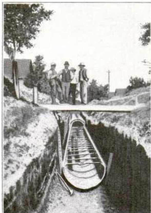
Collapsible Steel Forms in Place for Construction of Lower Half of Concrete Sewer
