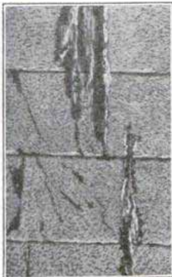
Filling Oozing through Outer Wall
