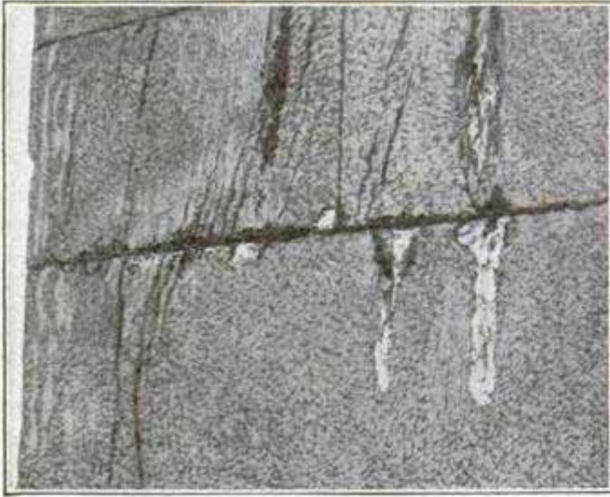
Cracks in Washington Monument Caused by Action of Alternating Heat and Cold, Dampness and Dryness
