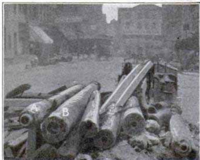
Wooden Water Mains Laid a Century Ago in New York and Still in Service in July of This Year
