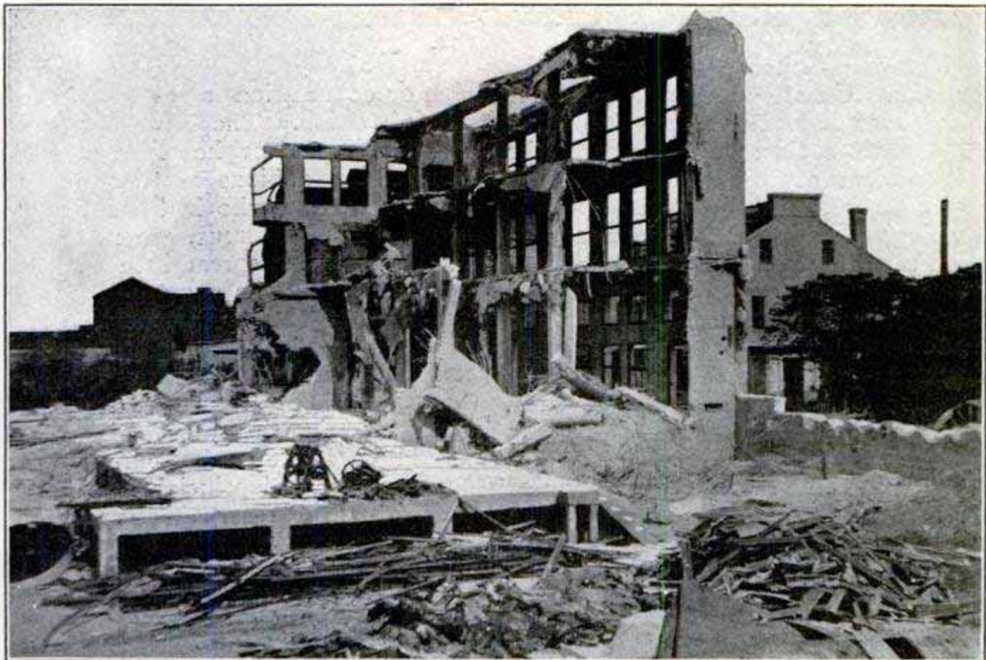
Concrete Flour Mill at New Orleans, Which was Wrecked with Dynamite at a Total Cost of $8,300 to Make Way for New Levee
