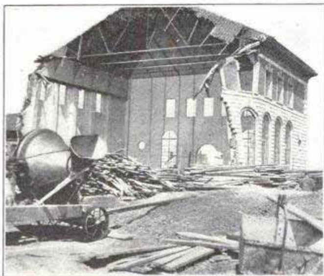
The New Buffalo Pumping House which Collapsed, Killing 15 Men and Injuring Many Others
