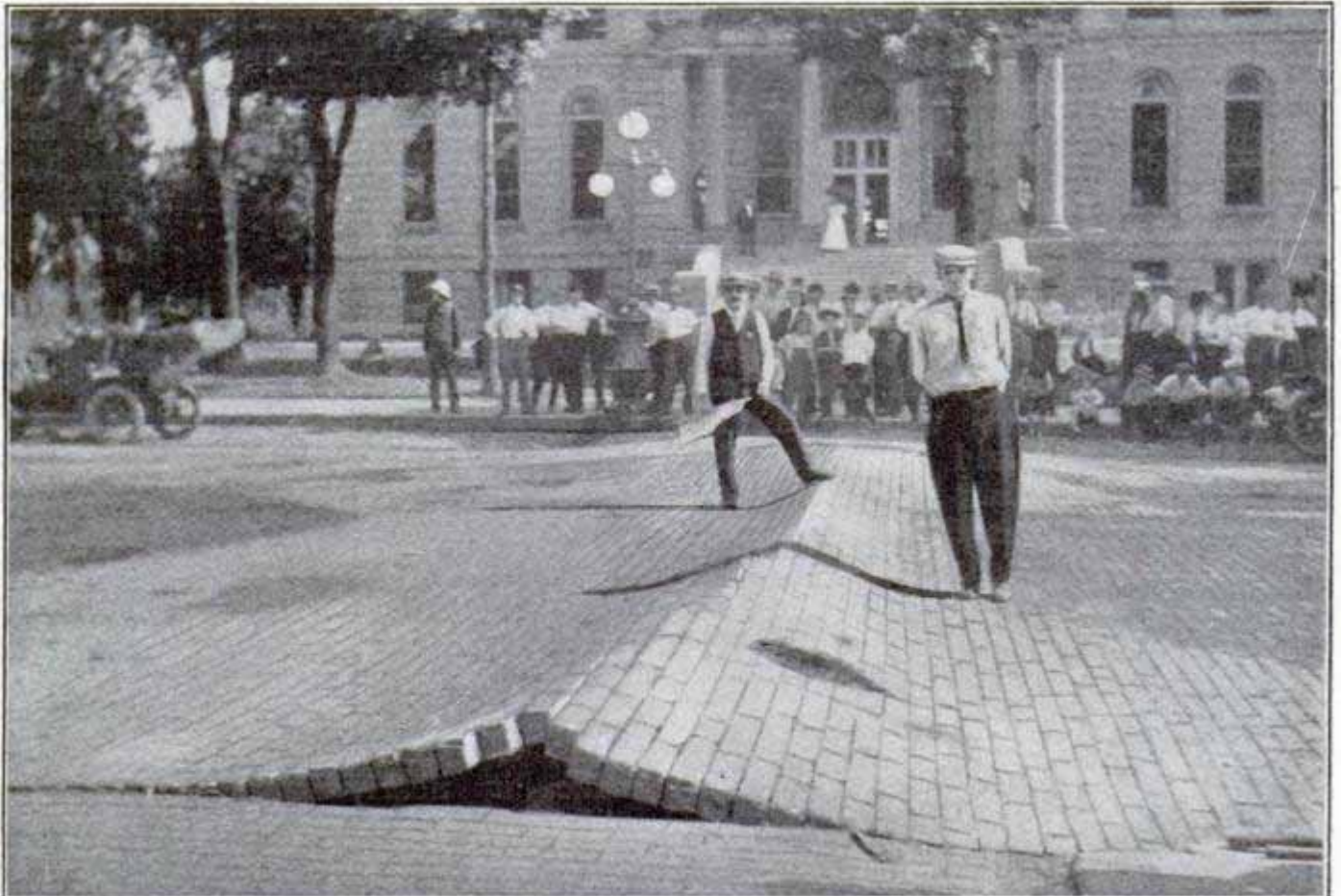
Section of the Pavement at Valparaiso, Indiana, Showing a Ridge Caused by the Intense Heat
