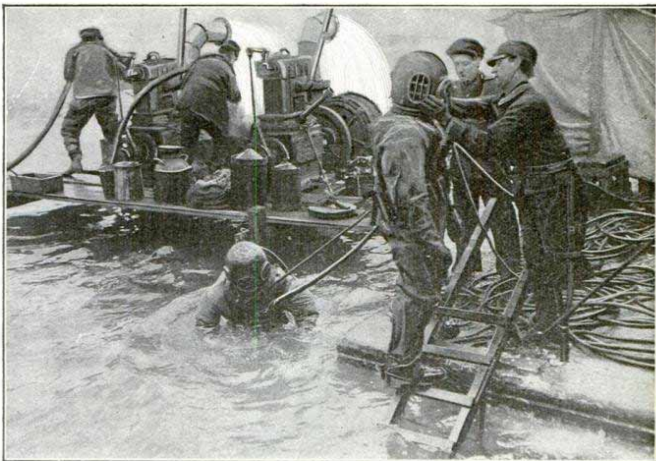
At Work in the Unsuccessful Attempt to Raise the Str. "W. C. Richardson," the Twin Pumps Emptying the Hull on the Left
