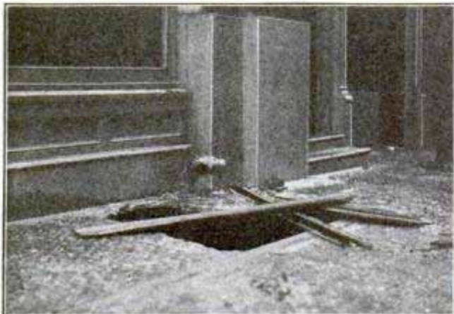
Hole Made in Iron and Glass Sidewalk by Bodies Falling from Top Floors of Building
