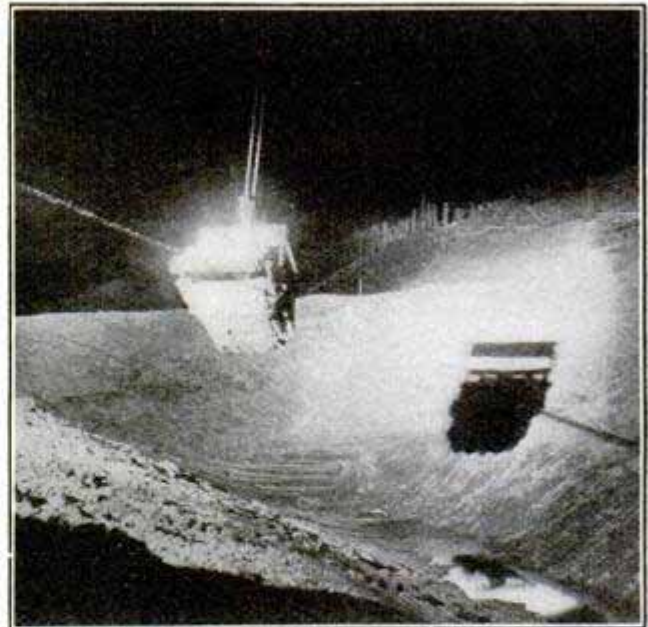
Excavation Bucket Used at Night with the Aid of Electric Light. Photograph Made 150 Ft. from Bucket, During Chicago Drainage Canal Work.
