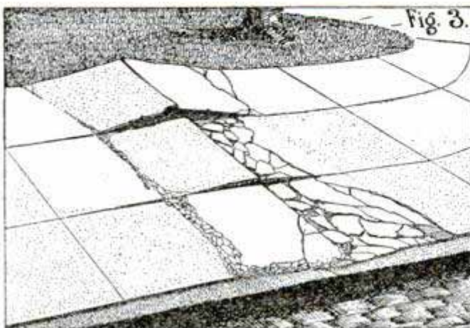
Bulging from Expansion
