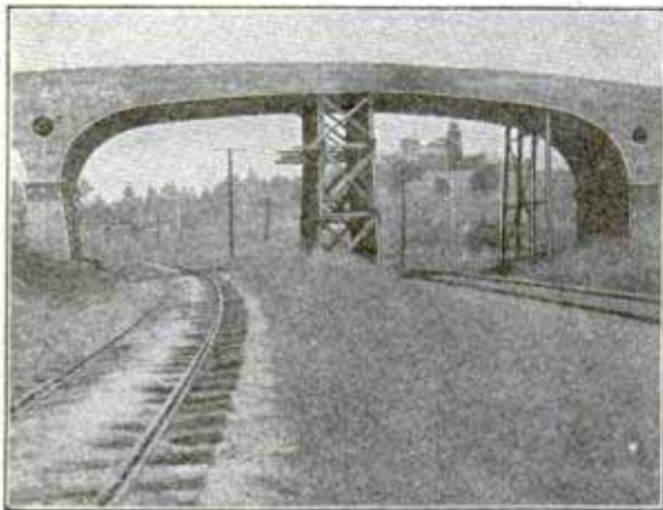
Arch That Failed
