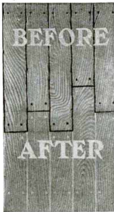
Section of flooring—cracks in lower portion filled with Johnson's Crack Filler.
