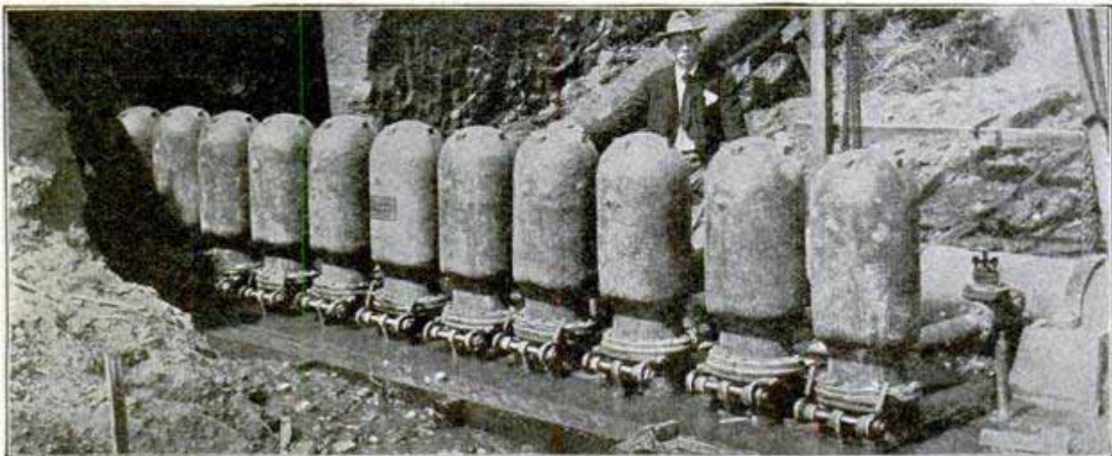
This Battery of 11 Rams Raises the Water 147 Ft.
