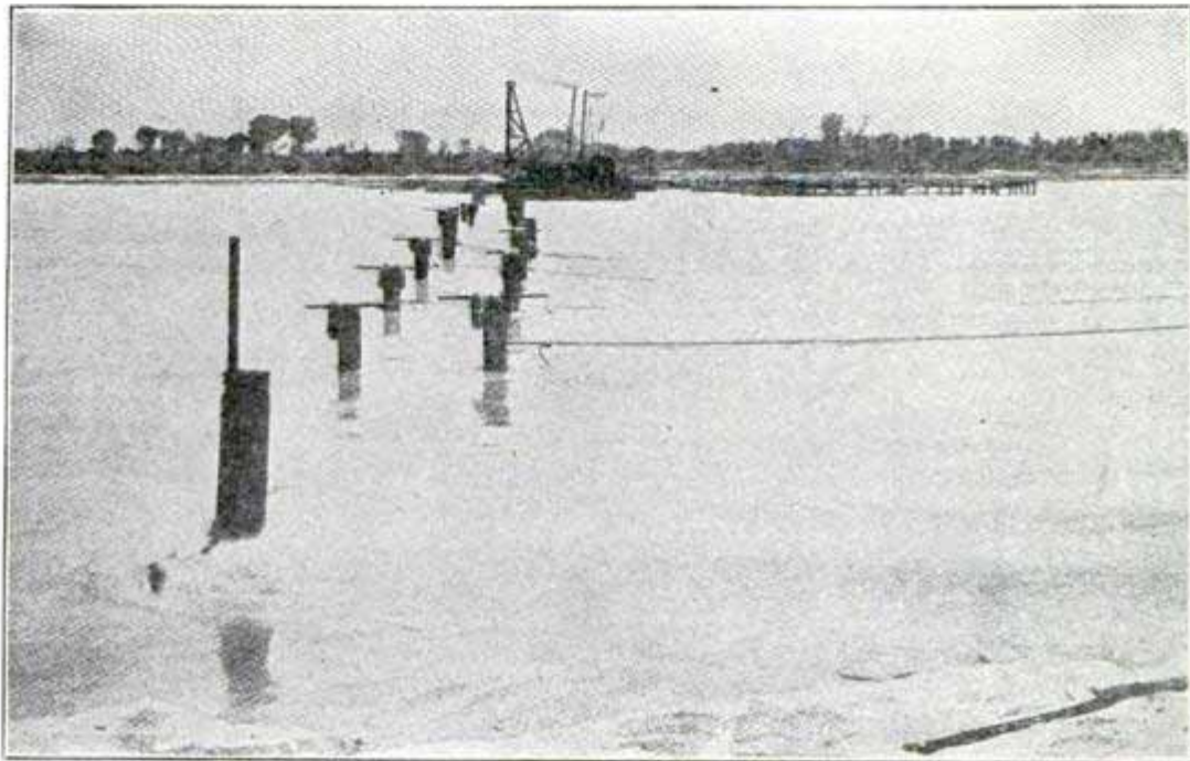
Piling for Railroad Bridge—Velocity of Water 12 Ft. Per Second. Photo by Lubken
