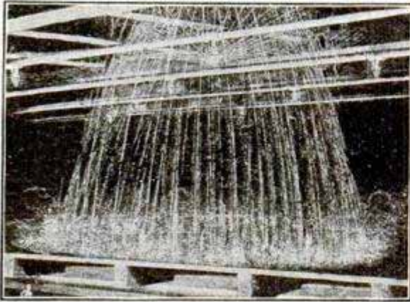
Sprinkler in Action
