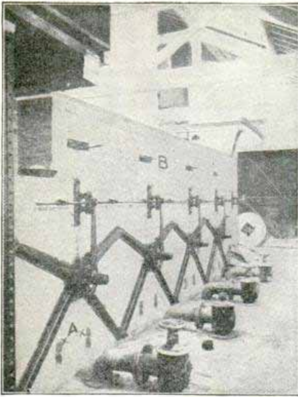
Fig. 2. Controlling Valves to Furnaces.
