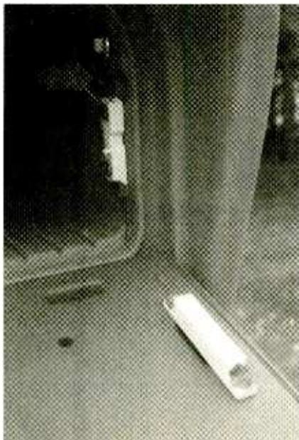
This closeup of the reed switch installation shows the liberal use of two-part epoxy to secure the switch and magnet in place.
